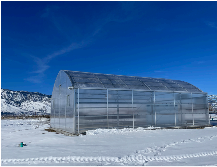
Above: Ioneer recently finished construction of a greenhouse near Gardnerville that is dedicated to research and conservation of Tiehm's buckwheat
